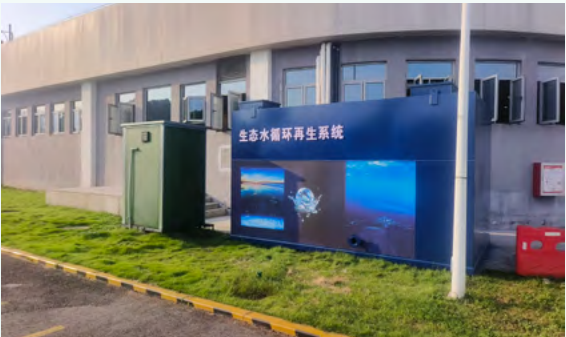
甬台温高速生态水循环再生系统 The ecological water recycling and reclamation system of Ningbo-Taizhou-Wenzhou Expressway
